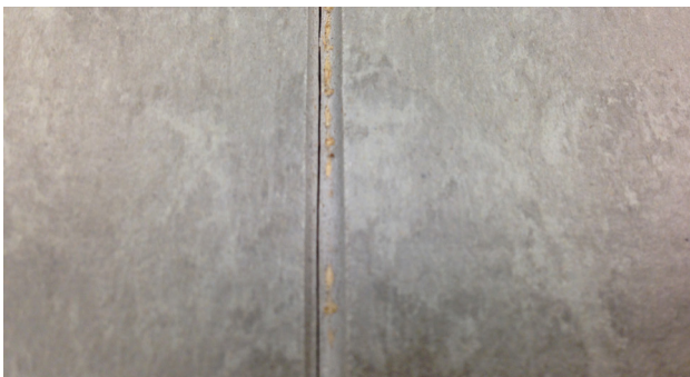
An off center groove will result in the weld rod pulling away from one sheet. This will result in a gap, or void, along one side of the seam that allows moisture and contamination to collect inside the seam and under the floorcovering.
