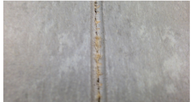
Example of properly grooved linoleum seam. Always groove deep enough to expose the jute backing.
