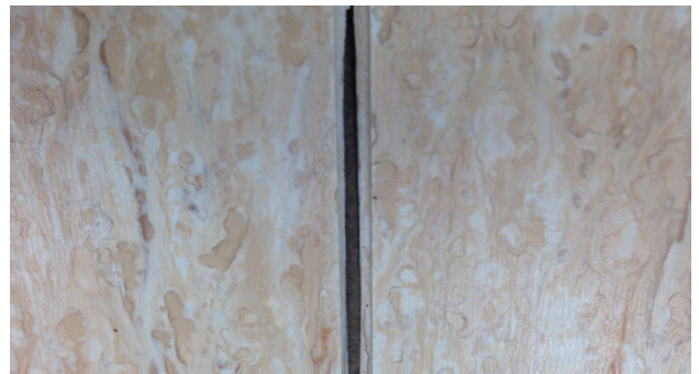
This seam has been grooved too deep and will result in seam failure.
