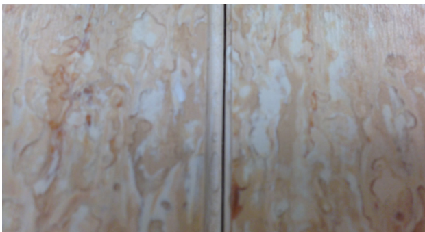
An off center groove will result in the weld rod pulling away from one sheet. This will result in a gap, or void, along one side of the seam that allows moisture and contamination to collect inside the seam and under the flooring.
