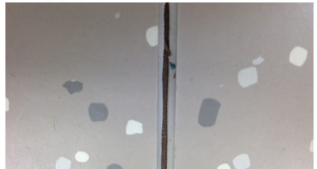
This seam has been grooved too deep and will result in seam failure.
