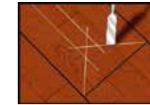
Picture 3: Remove the center section from the board. To be sure not to damage the neighbouring boards, use a chisel and manually extend the cut all to edges of neighbouring boards.
