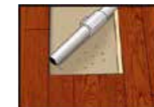
Picture 5: Vacuum carefully all wood dust and smaller wooden parts, to make area free and prepared for laying new board.
